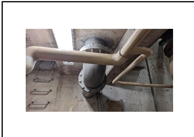
Photograph 11: Lead-containing grey paint observed on large diameter steel piping in Loc 4, pump room.
