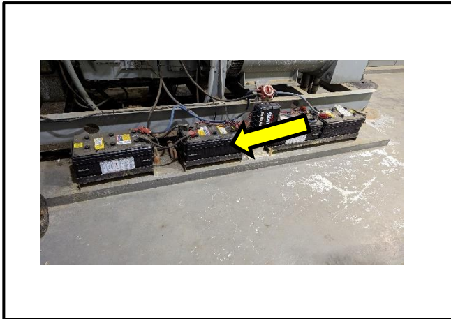
Photograph 13: Lead-acid batteries were observed connected to a backup generator in Loc 2, electrical room.
