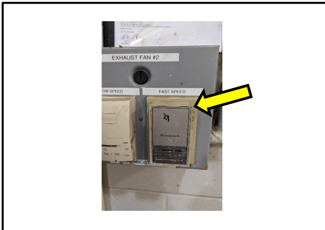
Photograph 15: A mercury vial was observed within a thermostat located on the north wall of Loc 2, electrical room.
