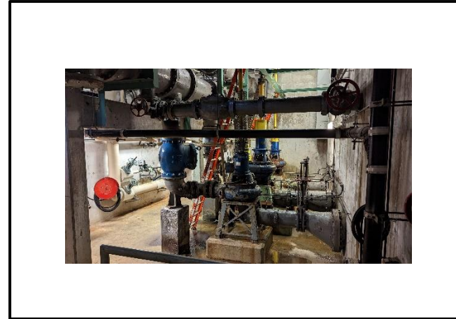
Photograph 6: View of Loc 4, pump room.
