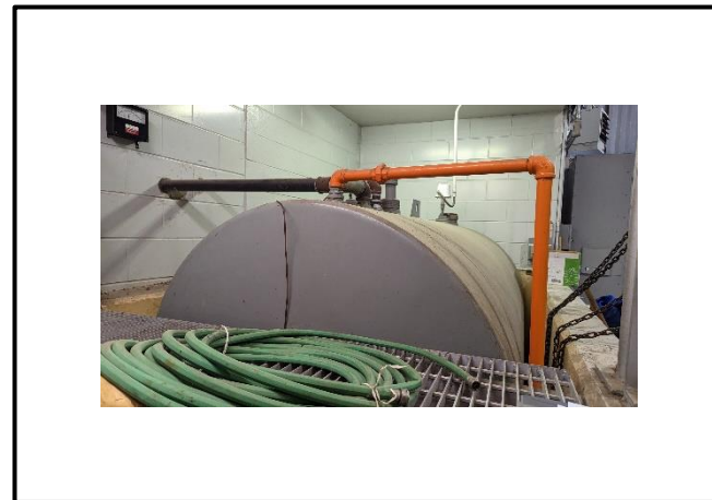
Photograph 16: A fuel storage tank was observed in Loc 2, electrical room.
