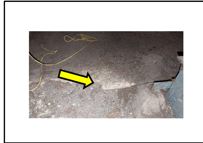
Photograph 10: Exposed asbestos-containing plaster observed in Loc 5, attic space.
