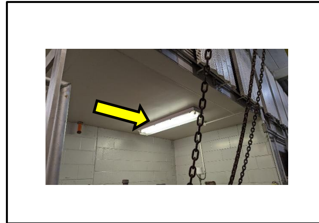
Photograph 14: Mercury vapour T8 fluorescent lamps were observed throughout the building.
