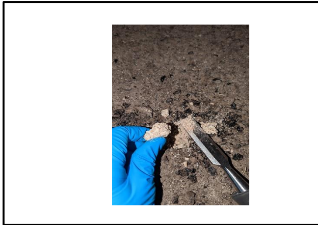
Photograph 9: View of asbestos-containing plaster concealed beneath tar and felt roofing in Loc 5, attic space.
